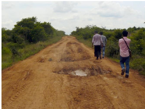
Photo 5: Very bad track in the settlement areas of Kampong Thom; for approx. 7 km around an hour of driving is needed
