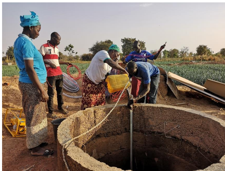
Figure 14: Women and men working together to install a solar pump in their market garden
