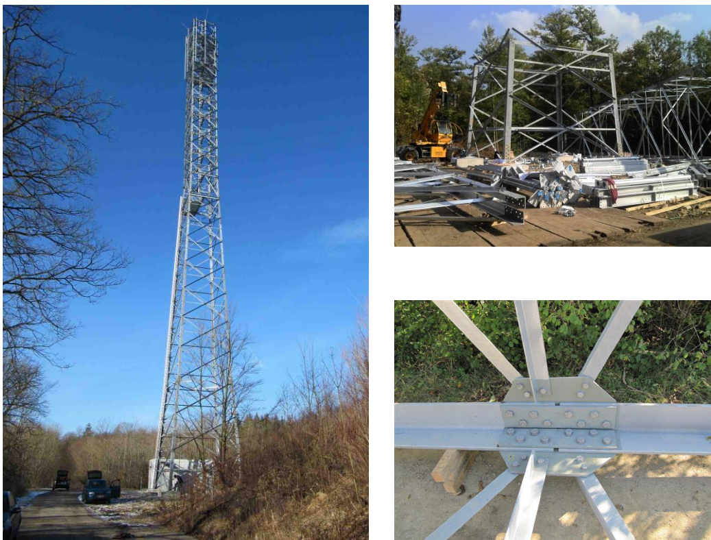
Figure 1 Radio masts with slip-resistant connections (photos: © CTeam)
