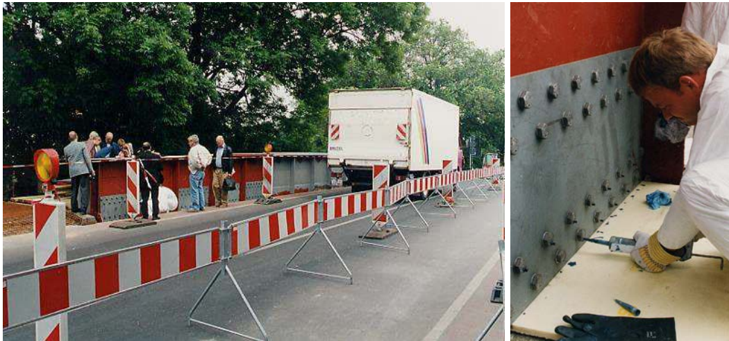
Figure 2.2: Injection bolts applied to repair an old heavily corroded riveted bridge Oranienburg (1994)
