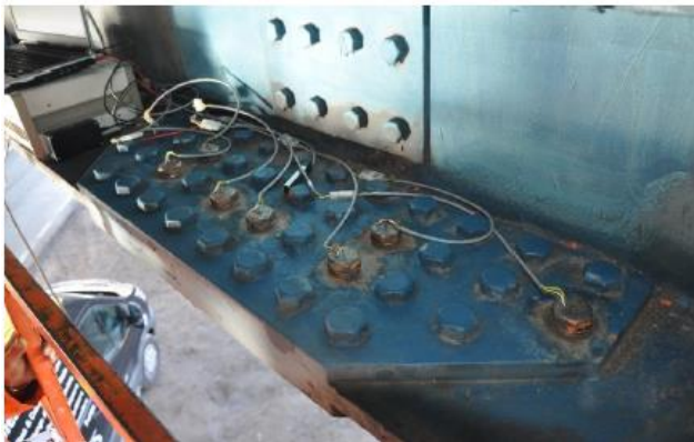
Top view of flange prior to the in-situ measurements. All 8 bolts on each side of the web that were instrumented were attached to data acquisition systems simultaneously. This way it was possible to monitor interaction between the bolts during (un)tightening.
