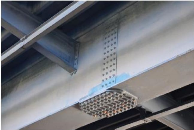
Overview of HCFG bolted splice joint in lower flange of the girder that was used to test the system. Bolt pattern consists of 4 \times 21 = 84 bolts. 16 of these were instrumented in situ.
