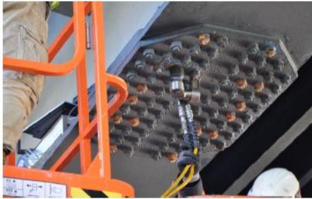
The new bolts were immediately pretensioned. The combined method was used to apply the preload
