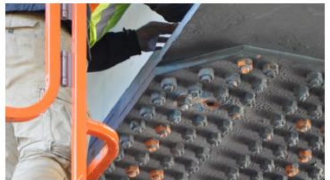
During the experiment the bridge was open for traffic. To ensure structural safety, directly after untightening a bolt, it was removed and replaced by a new bolt. This way the reduction of the resistance of the joint was restricted to only one bolt.
