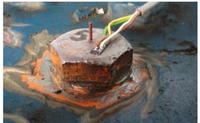
Prior to drilling of the hole the coating on/around the bolt head was removed. Picture shows bolt head with protruding stain gauge insertion pipe and glued on wire terminal.
