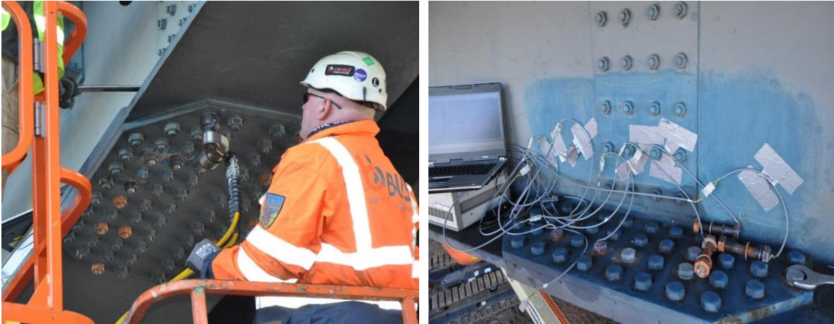
Figure 34 - Left: loosening of nut, right: removed bolts connected to terminal and laptop
