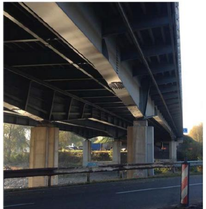
Main girders of the bridge. The girders are built-up sections with varying height and plate thickness of web and flanges. Steel grade S355. In the time the bridge was built faying surfaces of HSFG connections were coated by aluminium spray metallizing ('AL geschoopeerd').
