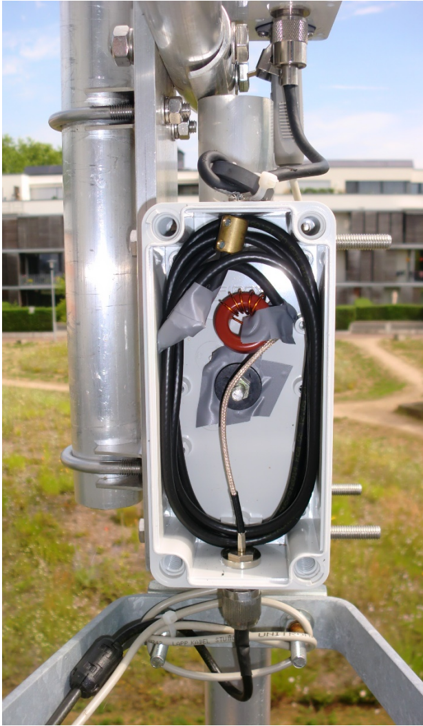
Fig.8 The realized matching circuit seen in a plastic box (open) mounted to the mast just below the feed point of the AMA82.
