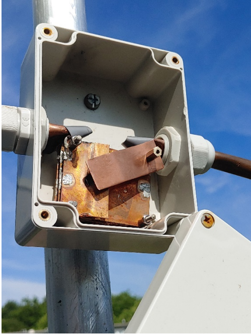
Fig. 7 The fixed capacitor between the ends of the small loop in the weatherproof housing on the mast of the AMA82.
